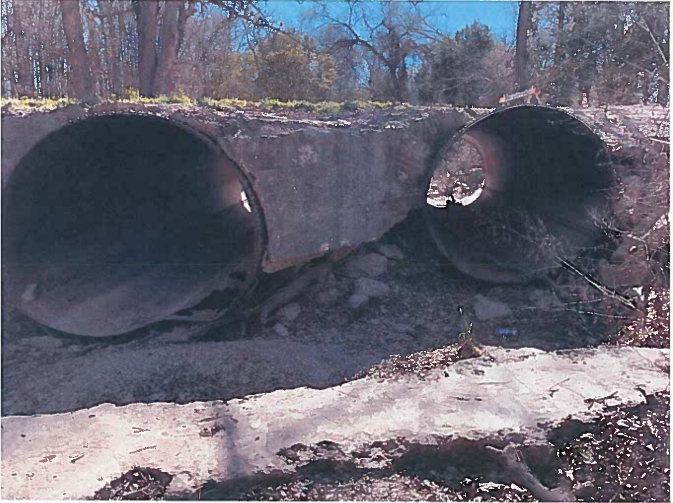
View from Downstream (note apparent hollow areas behind concrete and around pipes)
