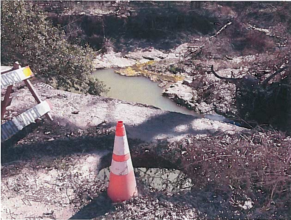
Looking Downstream (note hole in concrete driving surface)
